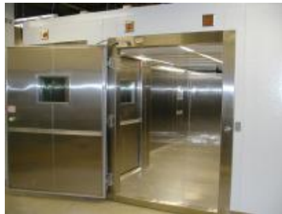
Hewlett Packard Dual Temperature/Humidity Room – controlled by Aromat PLC, includes temp/humid vs. time profile control and HMI
